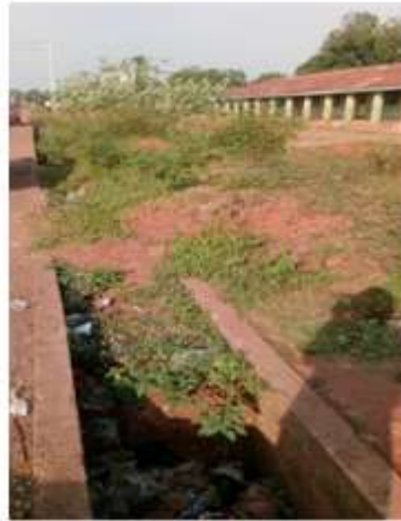
Plate 1: showing blocked drainage system.
